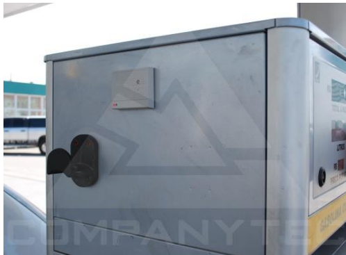
Figura 14 – Sensor IDF04 instalado
